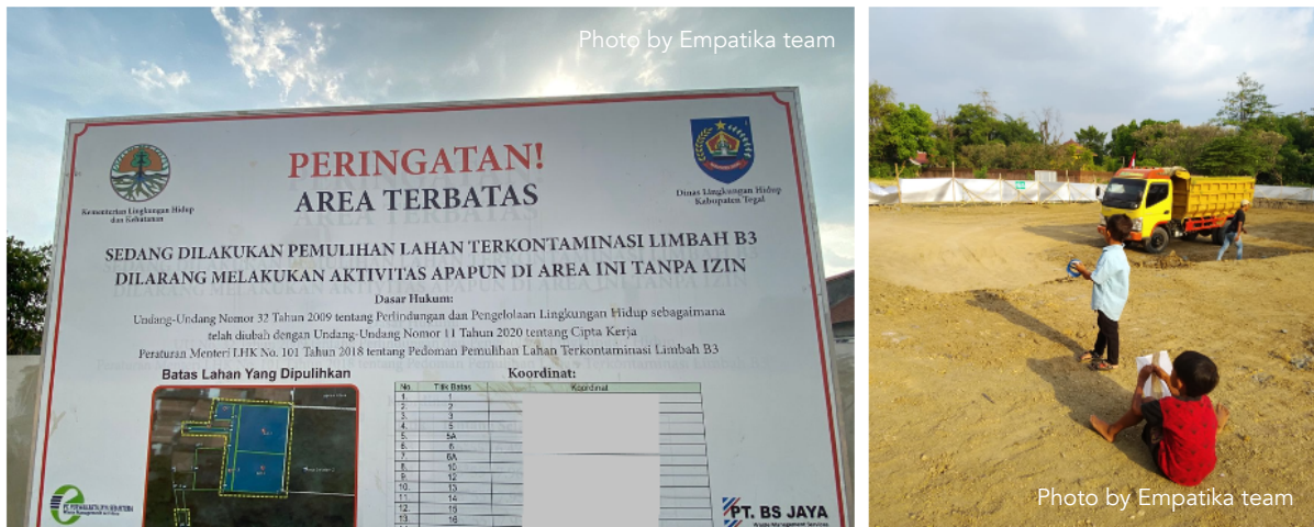
A waste field in Tegal village is being rehabilitated. It has a sign (left) warning people not to do any activities there, however it was not fenced off and children could access the area and play there.
